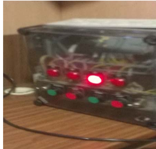
Fig. 11: Stage 3 of output generated on PLC.
