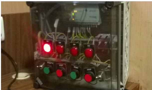
Fig. 9: Stage 1 of output generated on PLC.
